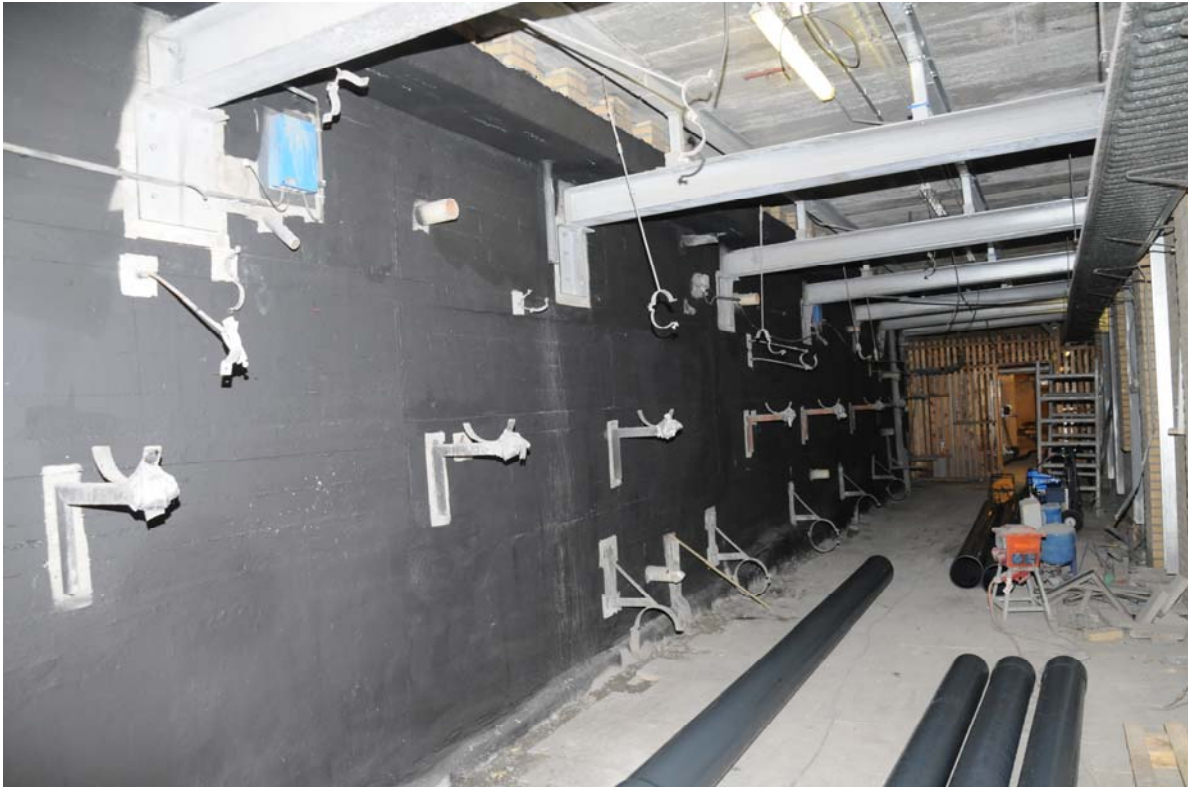
CAST 3+ Composite Anode installed on the outside walls of one of the swimming pools - overview
