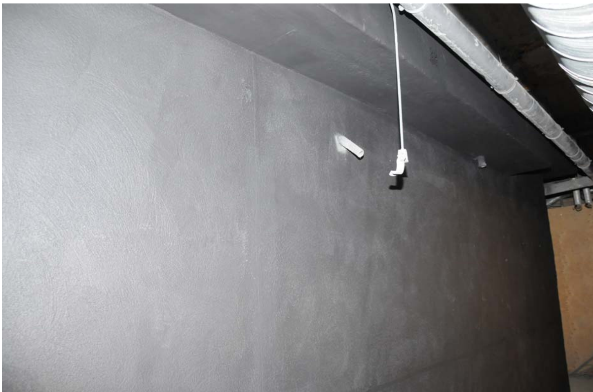
CAST 3+ Composite Anode installed on the outside walls of one of the swimming pools - close up view
