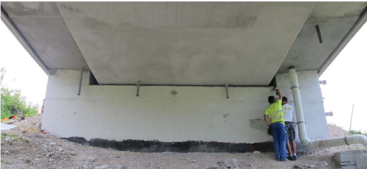
EZA on the abutment of the Alplgraben bridge after sand blasting (21 August 2012)
