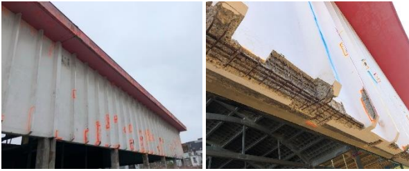
Fig. 15. Concrete damages due to carbonation
