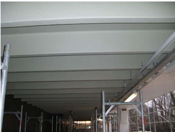
Fig. 5. CAS-T Composite Anode applied to concrete beams and soffits, covered with an elastic acrylic cover coating.
