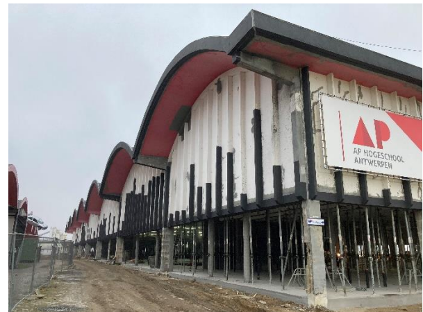
Fig. 17. Applied anode material (black conductive coating) on ribs, beams and roof elements
