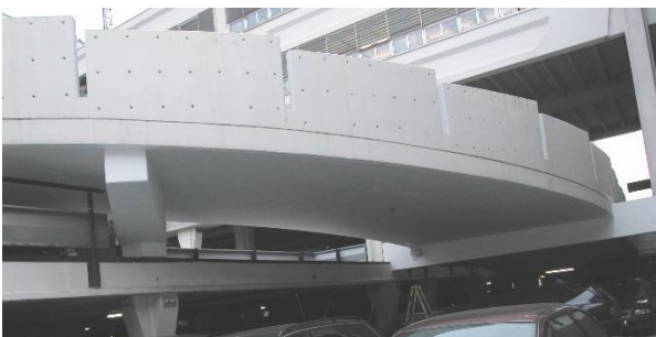
Fig. 6. CAS-T Composite Anode applied to beams and soffits, covered with an elastic acrylic cover coating.
