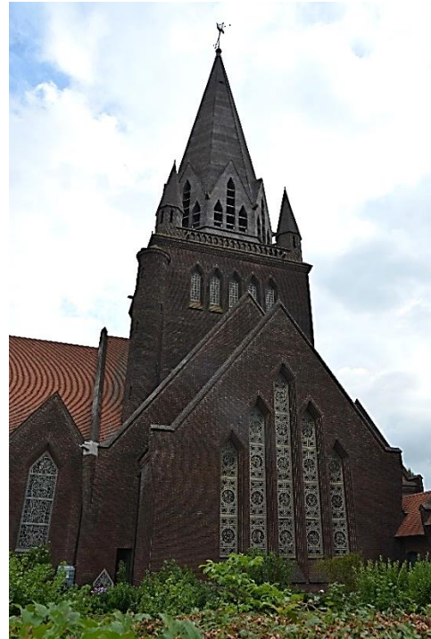
Fig. 8. Sint-Theodardus Church in Limburg, Belgium, elements protected with CAST Q Composite Anode, details see figure 9 below.
