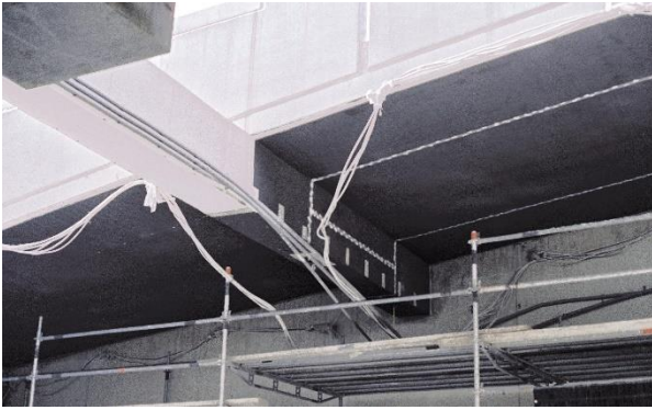
Fig. 3. Application of the CAS-T Composite Anode on the soffit of the drive-in ramp of the ORF parking garage
