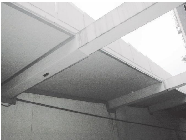
Fig. 4. CAS-T Composite Anode covered with a polyacrylic cover coat on the soffits and beams of the drive-in ramp to the ORF parking garage.
