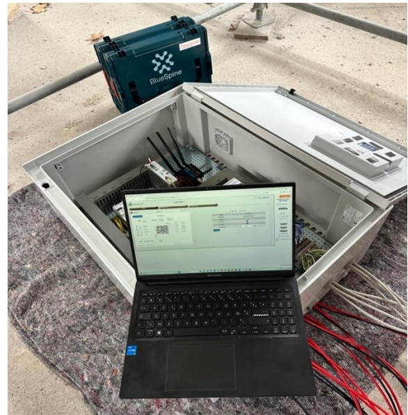
Fig. 37. Real-time data acquisition using an advanced automated monitoring system.
