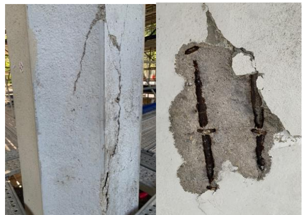
Fig. 31. Cracks and spalling due to corrosion of steel rebars initiated by carbonation of their concrete cover.
