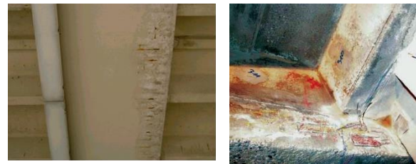
Fig. 2. Concrete damage caused by the steel reinforcement corrosion induced by the concrete cover carbonation.
