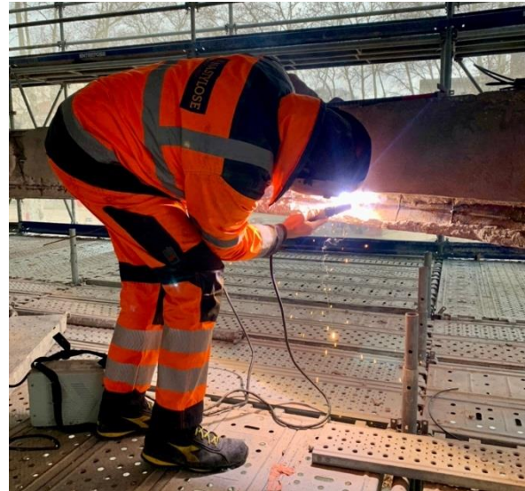
Fig. 33. Welding of the stirrups to an additional circular rebar to ensure steel continuity.
